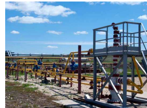
VM#1 wellhead and flow line
